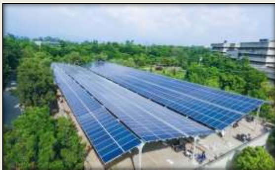
450 kWp Solar Plant at Two wheeler Parking at GMCH-32
